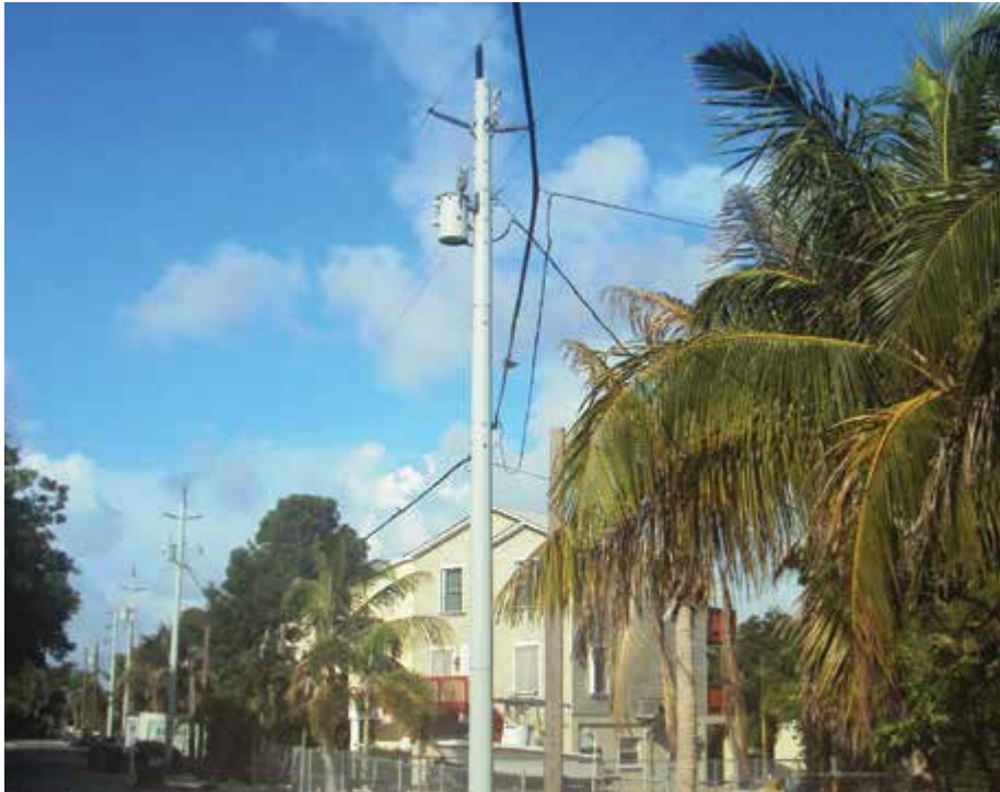
▶ Corrosive Environments & Coastal Areas
